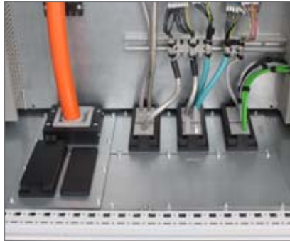
Cable routing via module plates in the base of a Rittal TS 8 enclosure. Mounting with icotek base plate KDR BMP.
